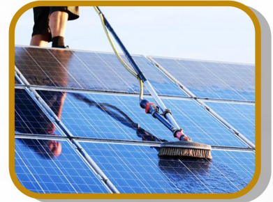
Annual Maintenance Service
