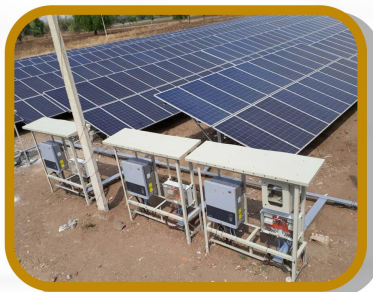
Solar Ground Mounted (Open Access)
